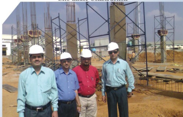
Inspecting the site (MGT Team)from left Mr.S.K. Dujari, Mr. N.G. Muramatti, Mr. Vijay Kumar & S.E.Dhand
